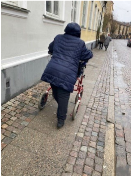
Figure 3: The walkway has a steep side slope, putting users in danger of falling, especially when using a walker or wheelchair.
